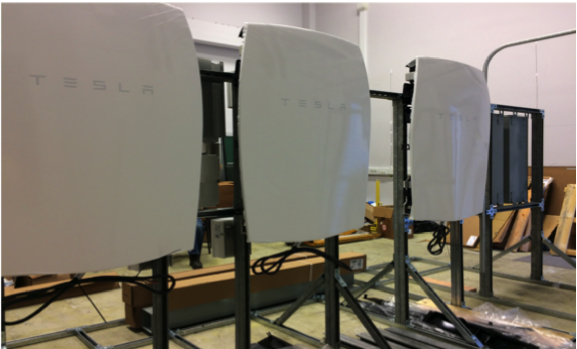
Figure 6 - Tesla PowerWall battery storage devices located at LBNL's FlexGRID facility.
