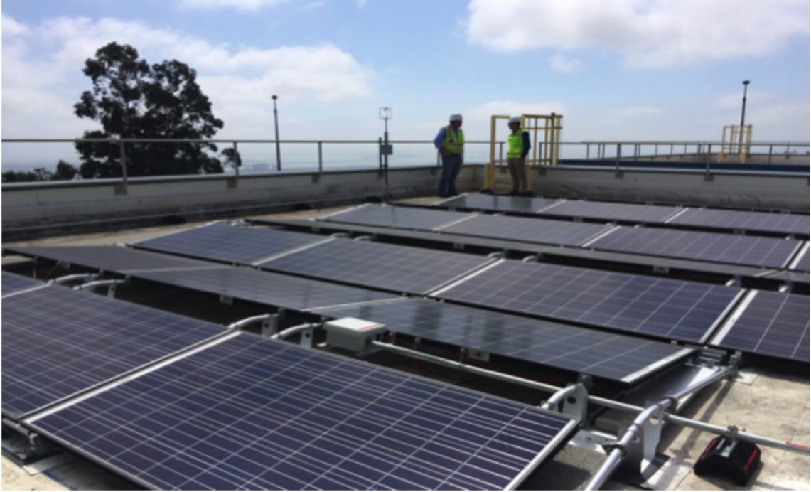
Figure 5 - Rooftop photovoltaic systems located at LBNL's FlexGRID facility.
